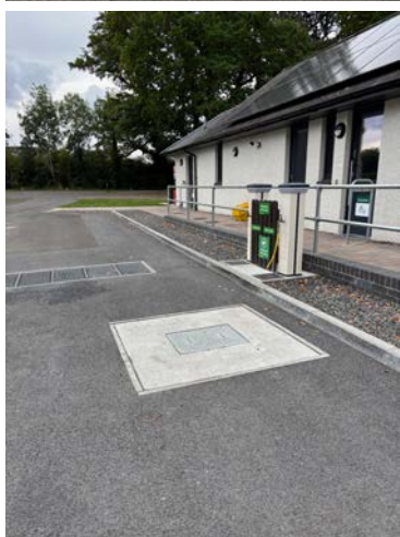
MHSP at Toilet Block B
