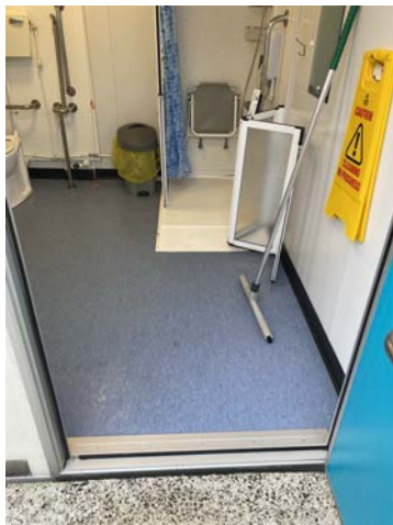
The entrance into the cubicle
